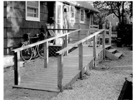
Ramp with stairs placed too close to the ramp and back door.
