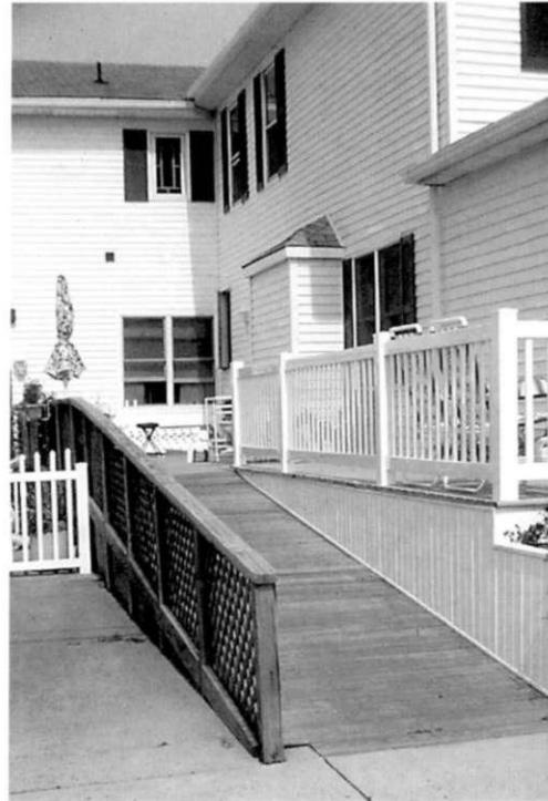
An attractive ramp (but it is missing a handrail on the right side).
