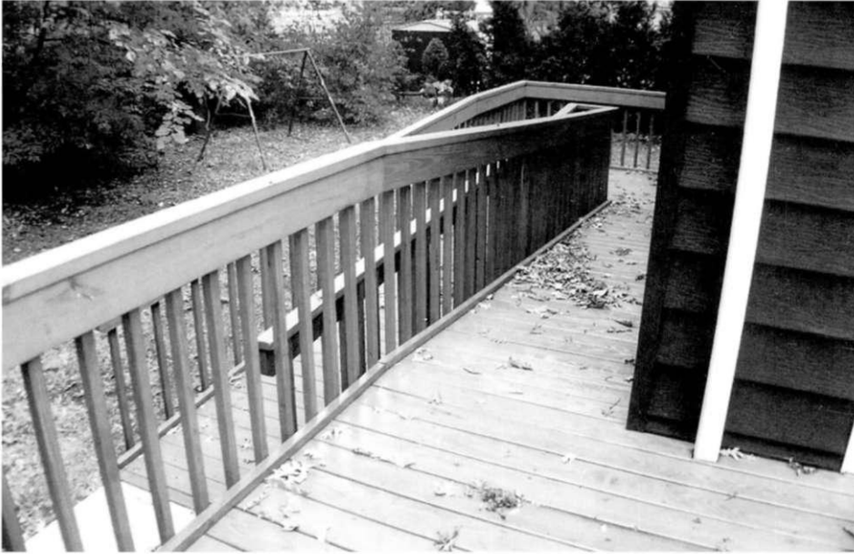
Ramp with double handrails and two-inch bottom ledge to prevent caster wheels from rolling off the edge.
