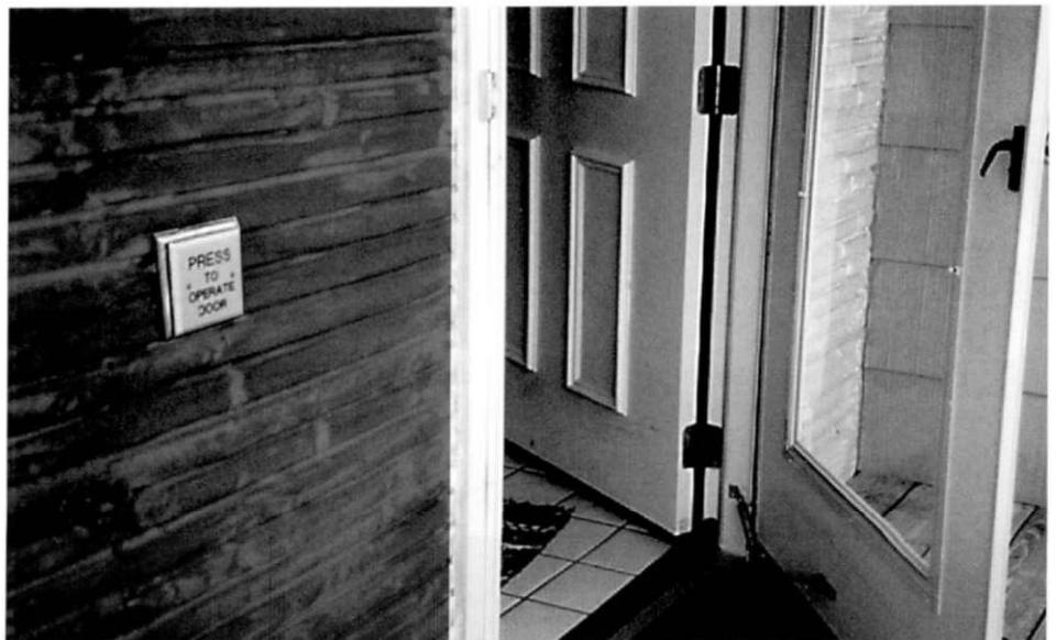
Push-plate power-assist door opener.
