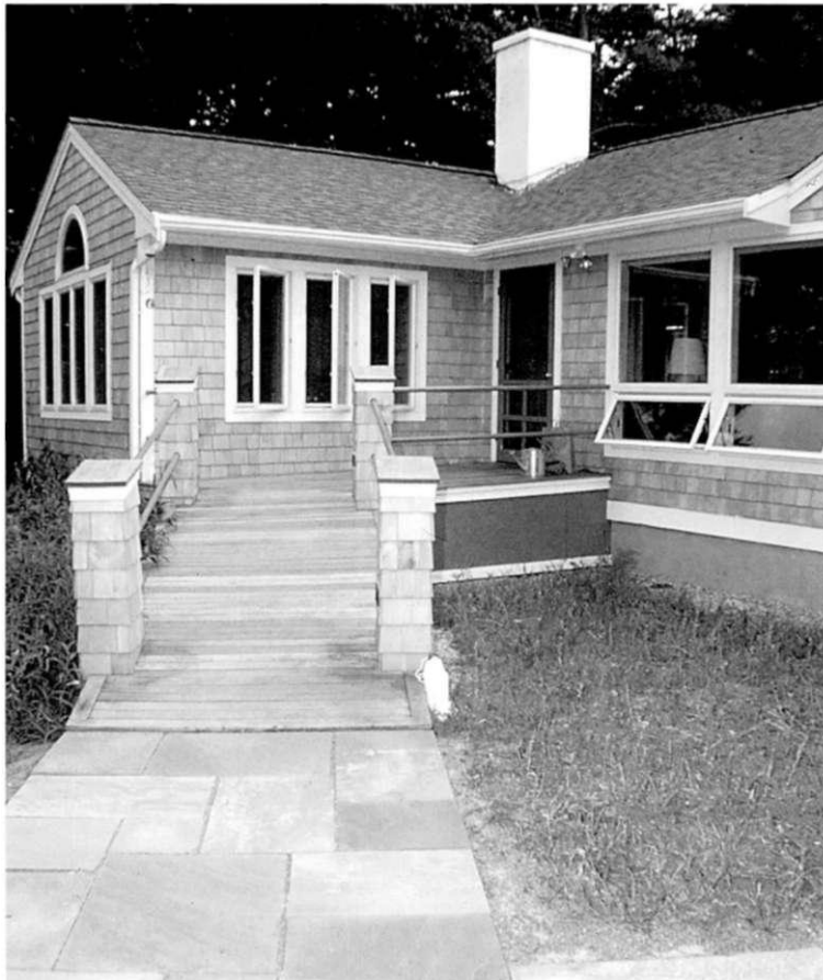
Attractive ramp but it is missing the ledge and handrail extensions.
