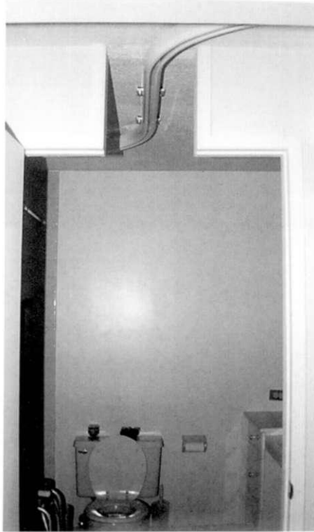
Header over door is partially removed to make room for overhead lift track.
